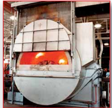
Barrel Melting Furnace
